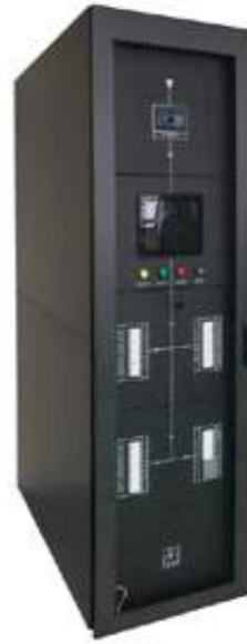
Precision Distribution Cabinet
